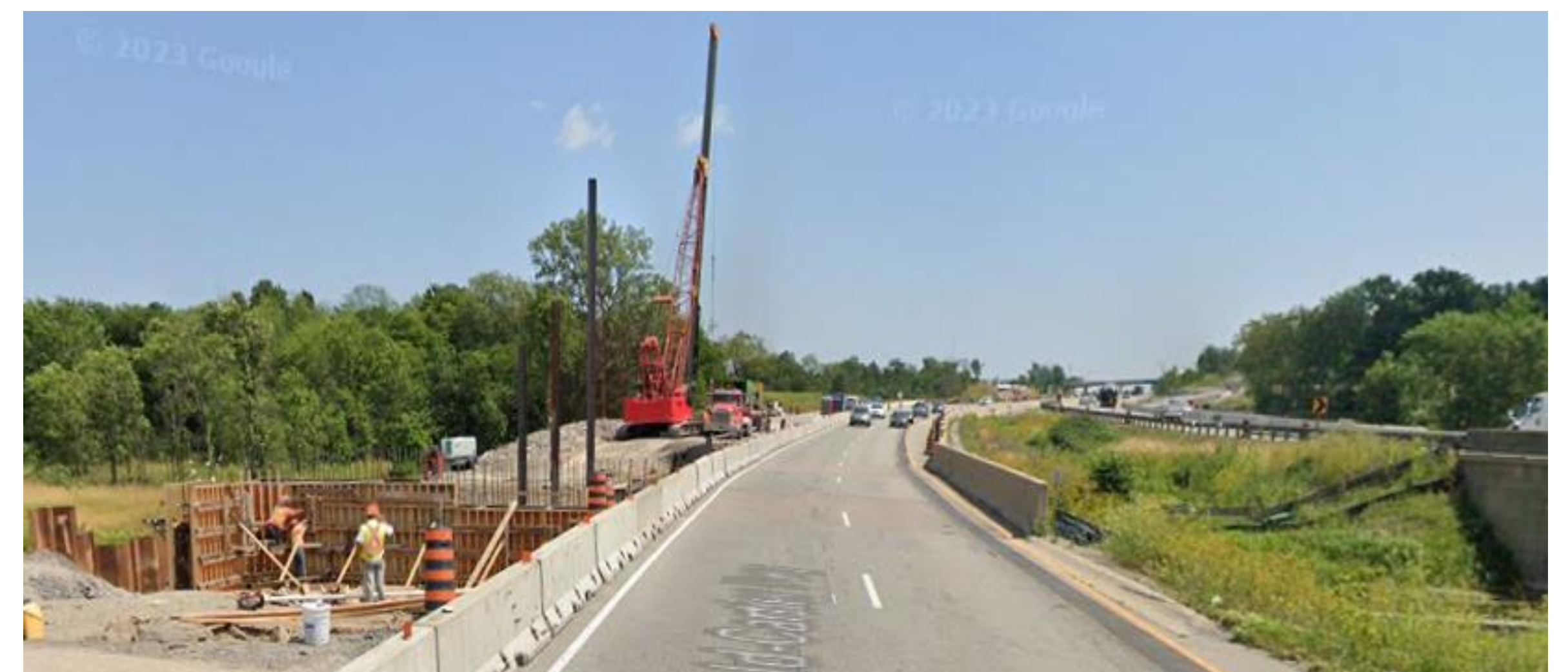
Figure 2: Example staged bridge replacement. East view of the recent staged replacement at WB Collins Creek (Contract 2018-4011) ( Preferred ).
